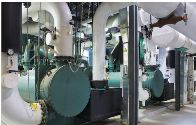
MannKind Corporation: centrifugal chillers and distribution piping in the CUB.
