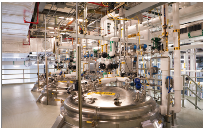
Biogen Idec: bioreactor buffer tank.
