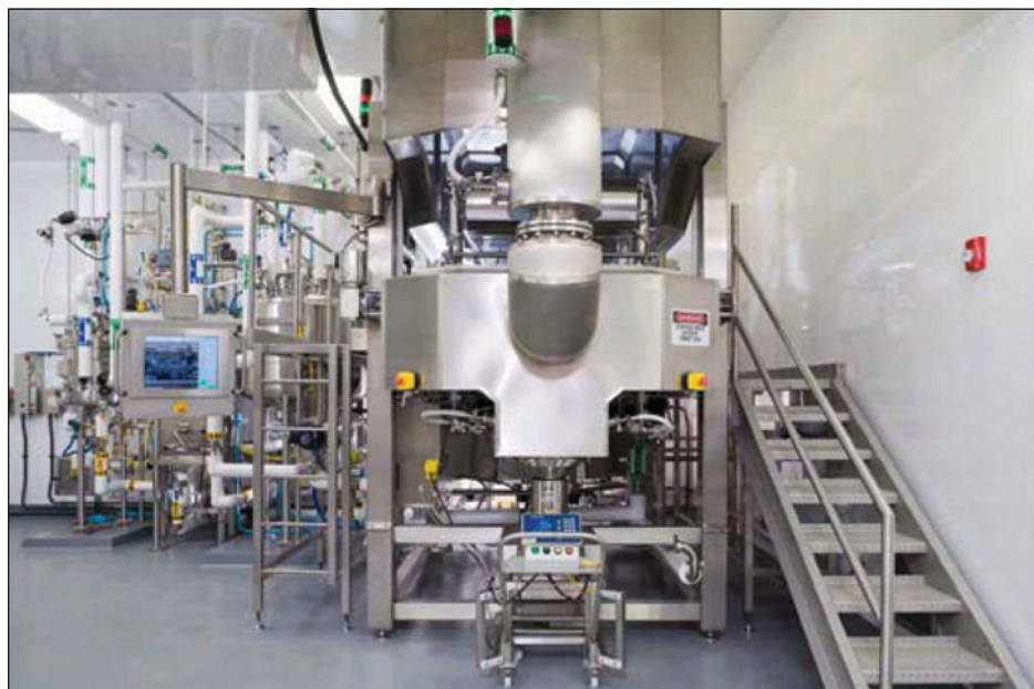
Cryopelletizer with the top section raised for inspection.
